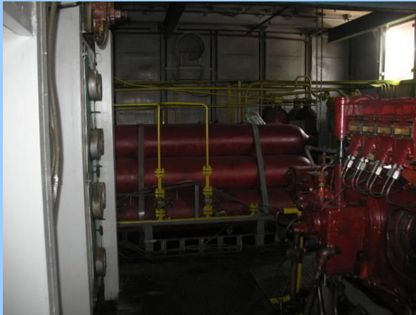
CNG Storage at a station in the Marneuli Municipality, Village of Jandara
