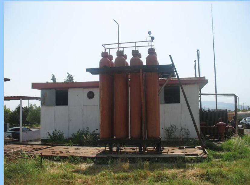
CNG Storage at a station in the Zestaphoni Municipality, Village of Argveta
